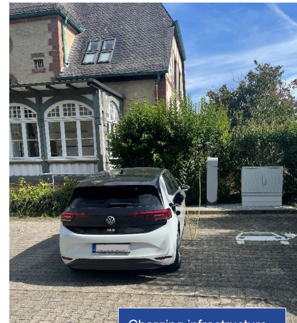
Charging infrastructure District Court Fritzlar
