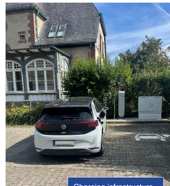
Charging infrastructure District Court Fritzlar
